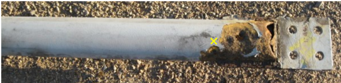
Thickness test location 22 for corroded members
