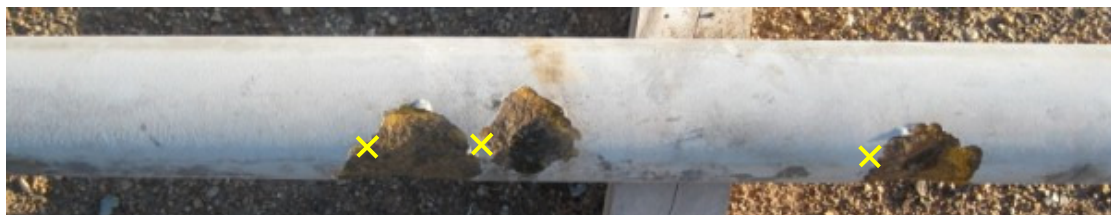
Thickness test location 4 to 6 for corroded members
