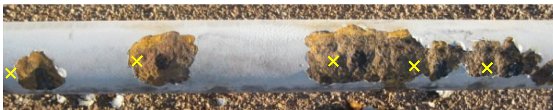
Thickness test location 7 to 11 for corroded members
