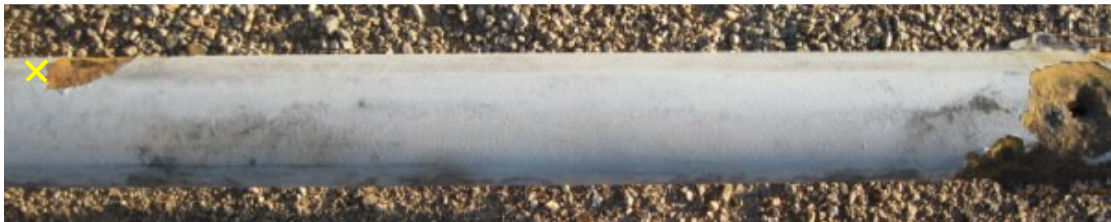
Thickness test location 21 for corroded members
