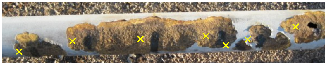
Thickness test location 13 to 19 for corroded members
