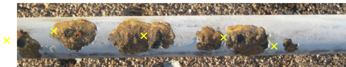
Thickness test location 8 to 12 for corroded members
