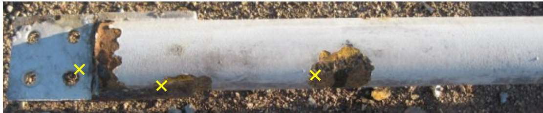
Thickness test location 1 to 3 for corroded members
