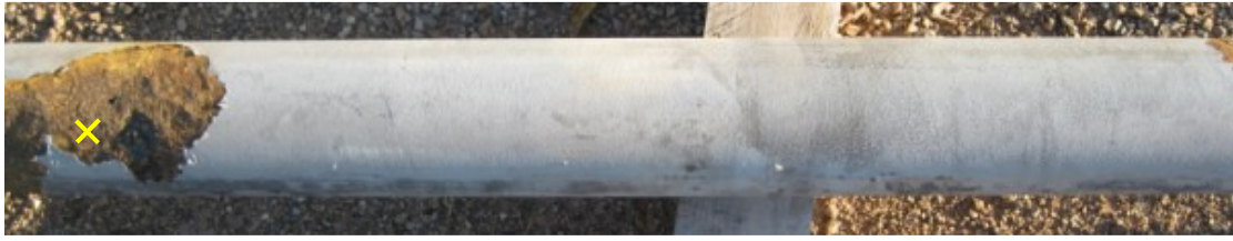
Thickness test location 20 for corroded members
